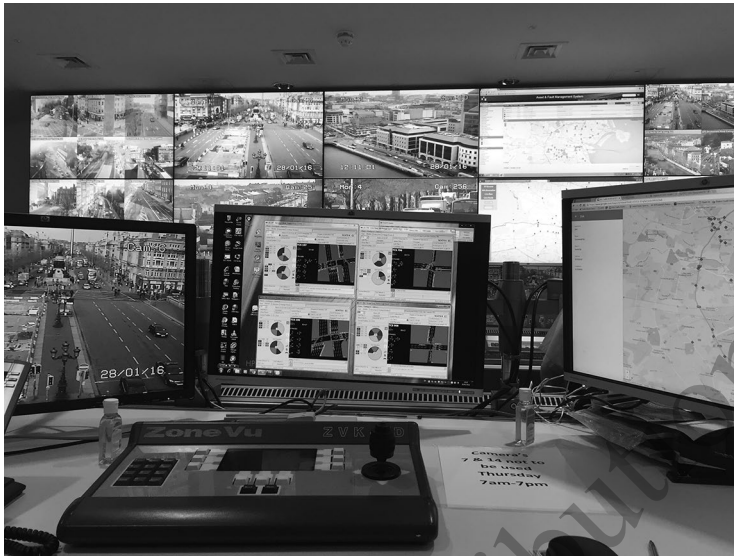
FIGURE 6.1 Part of the traffic control room in Dublin.
